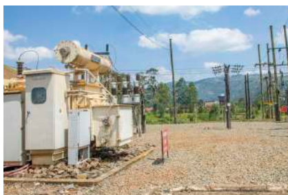
Kabale Central Substation From 2.5 MVA to 5MVA
