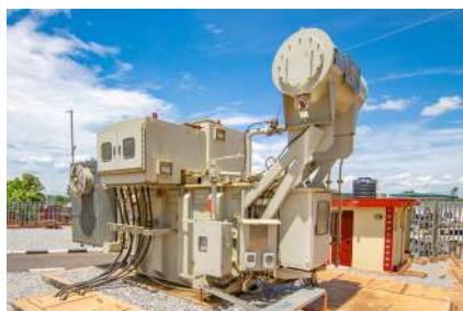
Kakiri Substation From 10/14MVA to 2 x10/14MVA
