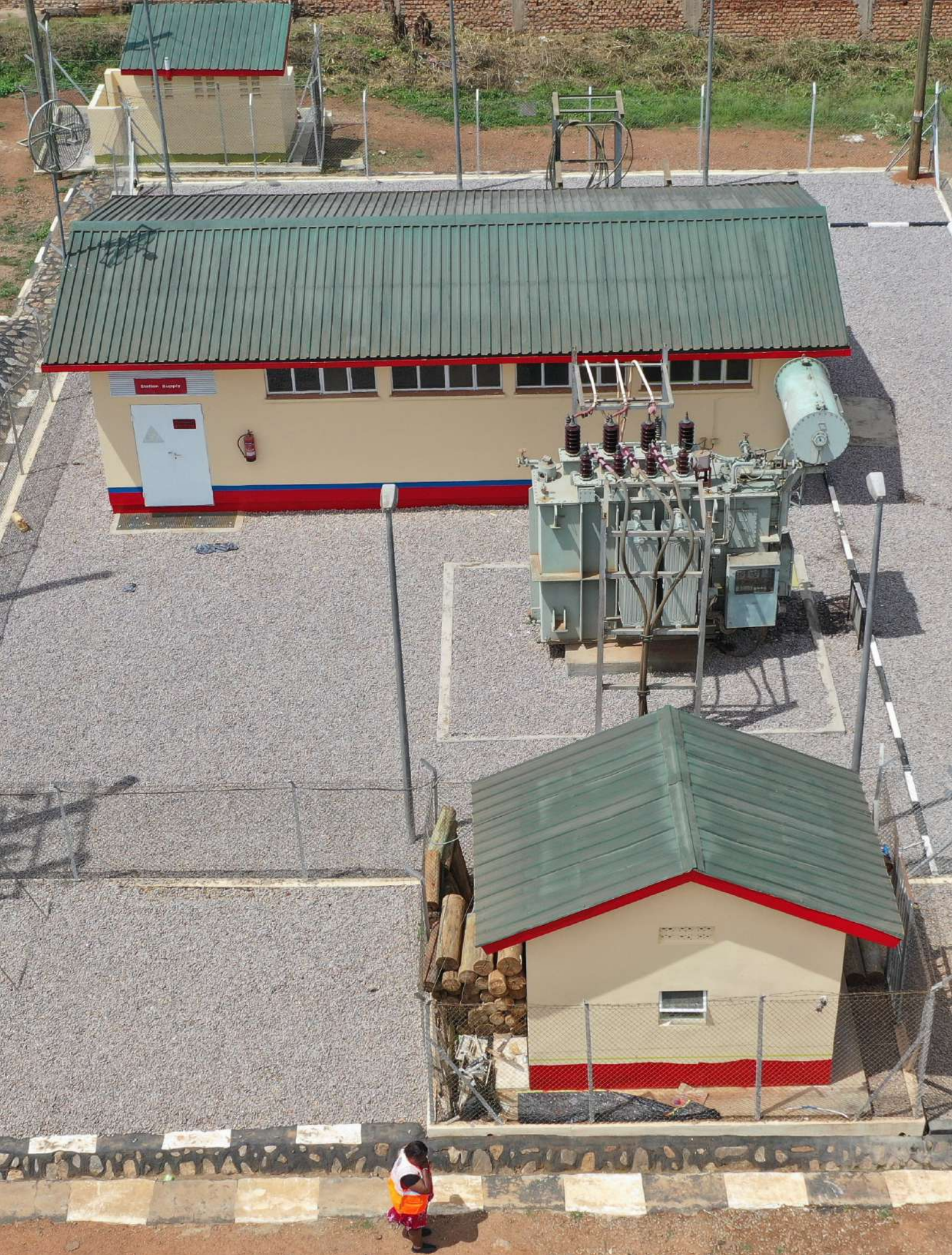
Masaka Substation 33/11 kV
