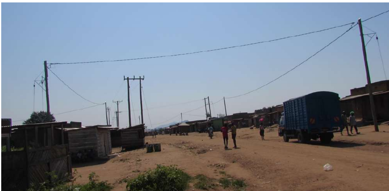
Lazebu Trading Center in WENRECo concession lacking access due to wayleaves
